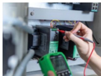
Industrial Automation & Control
