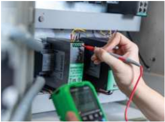
Industrial Automation & Control
